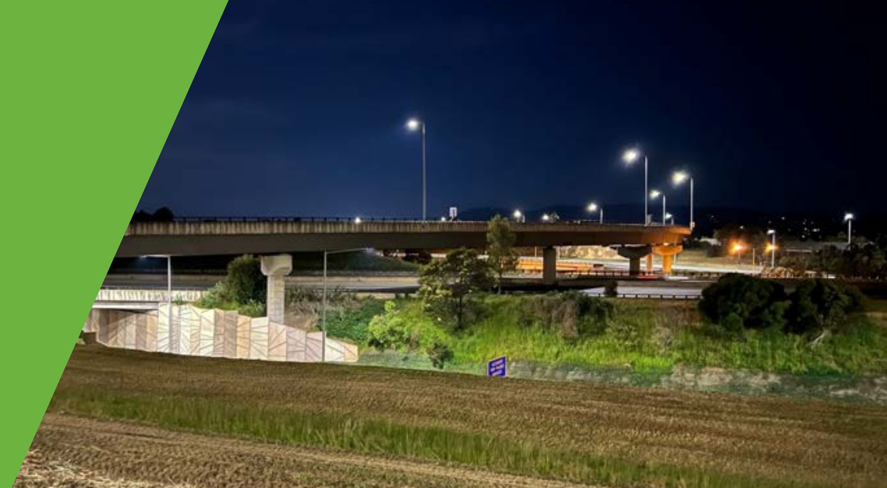
New LED luminaires at the Monash Freeway Interchange. Note the old HPS luminaires in the centre-right of the image, which have since been replaced.
